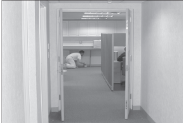
Construction workers near completion of the final phase of the build-out. This main row of cubicles is now the home of the Foreign Pharmacy department and Office Services.
